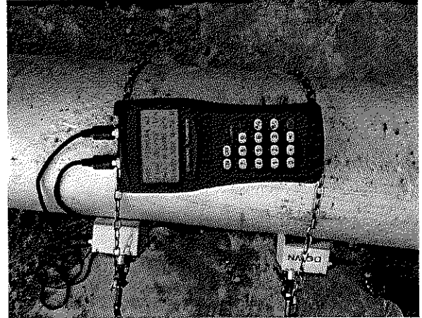
Plate 8 Flow measurement in supply pipe with ultrasonic flowmeter
